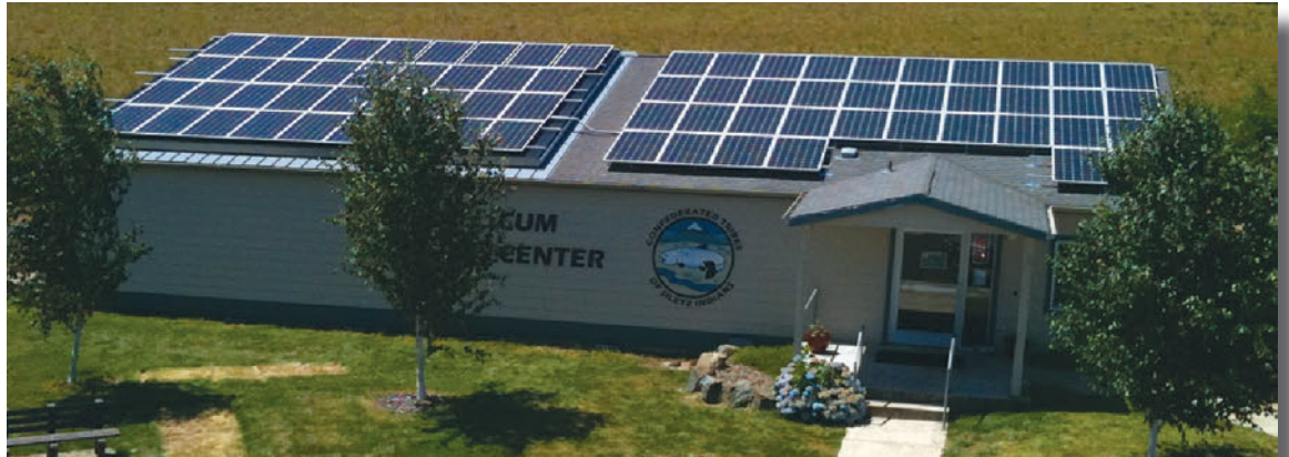
Solar panels on the roof of the Tillicum Fitness Center in Siletz
