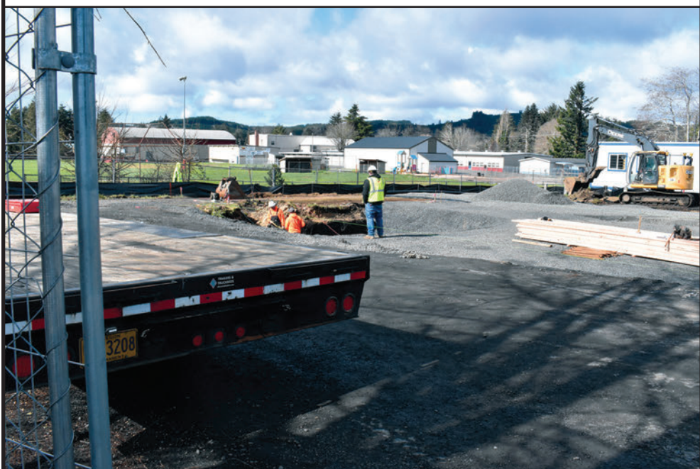
Construction continues in snowy weather (above) and sunshine (below) at the site of the new pharmacy building in Siletz.
